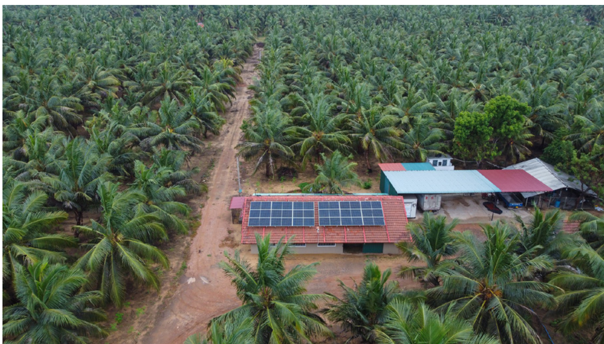
Solar panels installed at an agribusiness in Sri Lanka power a containerized cold storage room. Photo: UNDP Sri Lanka
