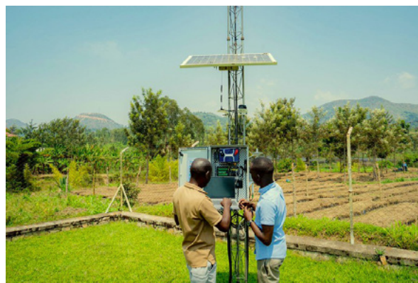
A solar powered early warning system in Rwanda. Photo: UNDP Rwanda
