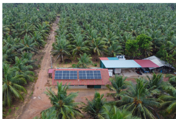
Solar panels installed at an agribusiness in Sri Lanka power a containerized cold storage room. Photo: UNDP Sri Lanka
