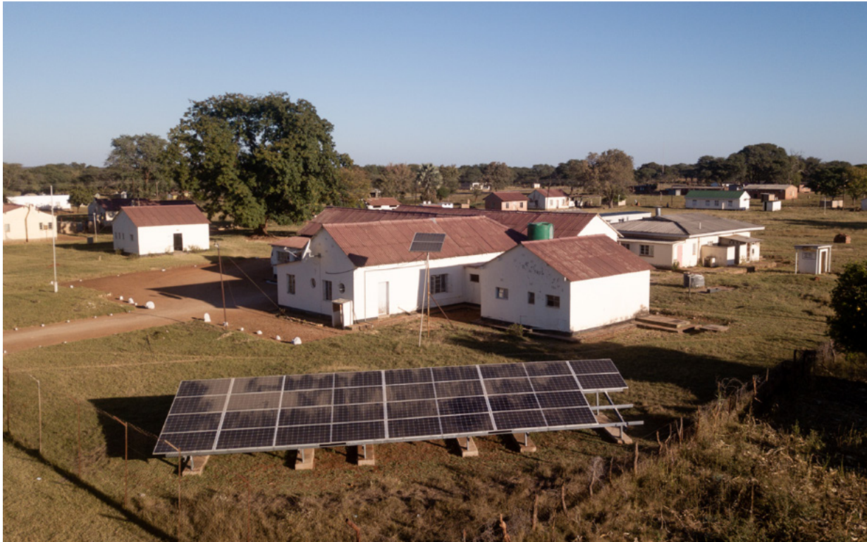
An installation in Zimbabwe as part of UNDP's Solar for Health programme.
