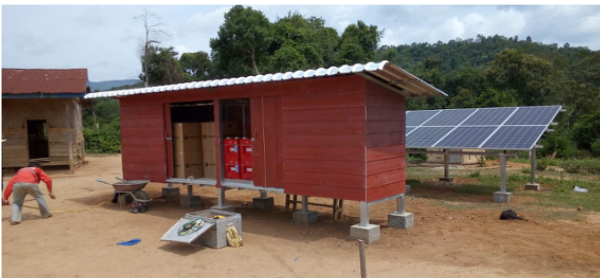
Figure 7: The Power-Hub as a central location for the energy infrastructure
