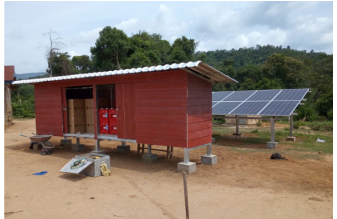
Figure 12: The Power-Hub as central place for the energy infrastructure
