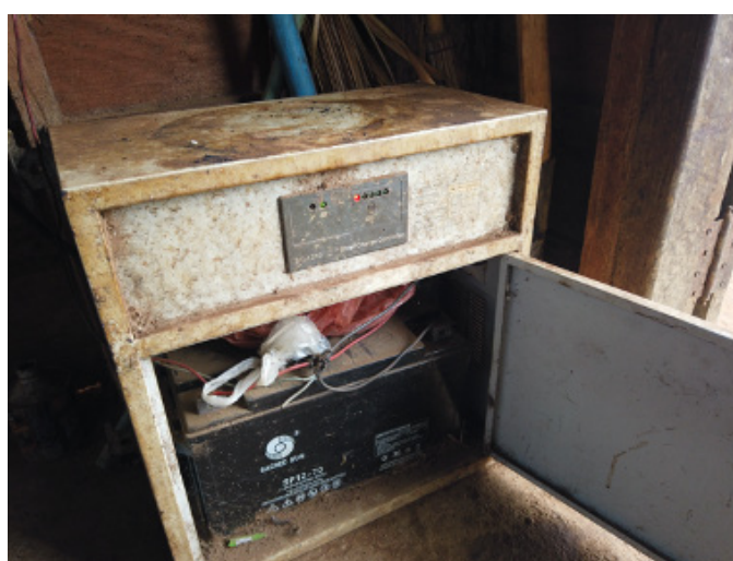
Figure 4: Old solar home system in Kobong
