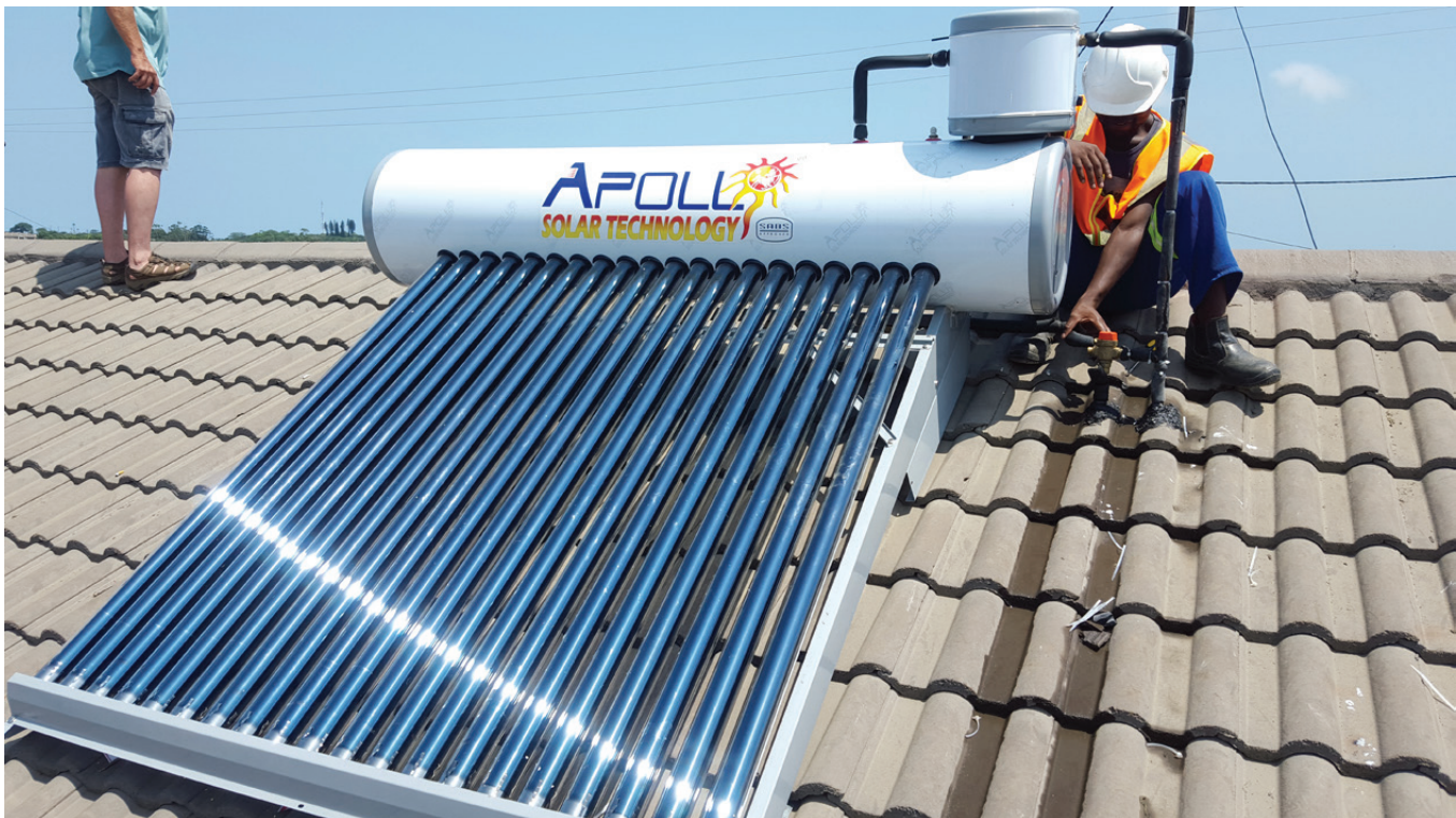
Solar water heaters save electricity and money – here installed on Groutville Care Homes in KwaDukuza, South Africa, as a pilot project implemented by Urban-LEDS
